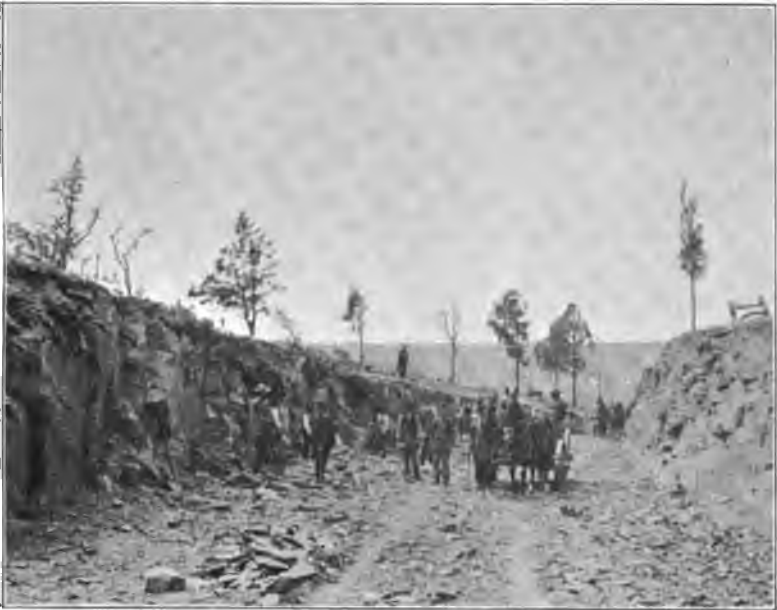
Marshall's Corner and Woodsville road, Mercer Co., working on 15-foot rock cut, during construction.
